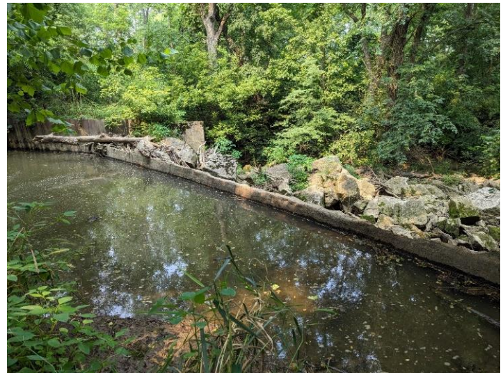
Photo: Looking N.E. at Bloody Run Weir, July 2023 Water was heard and observed leaking through weir below the waterline
