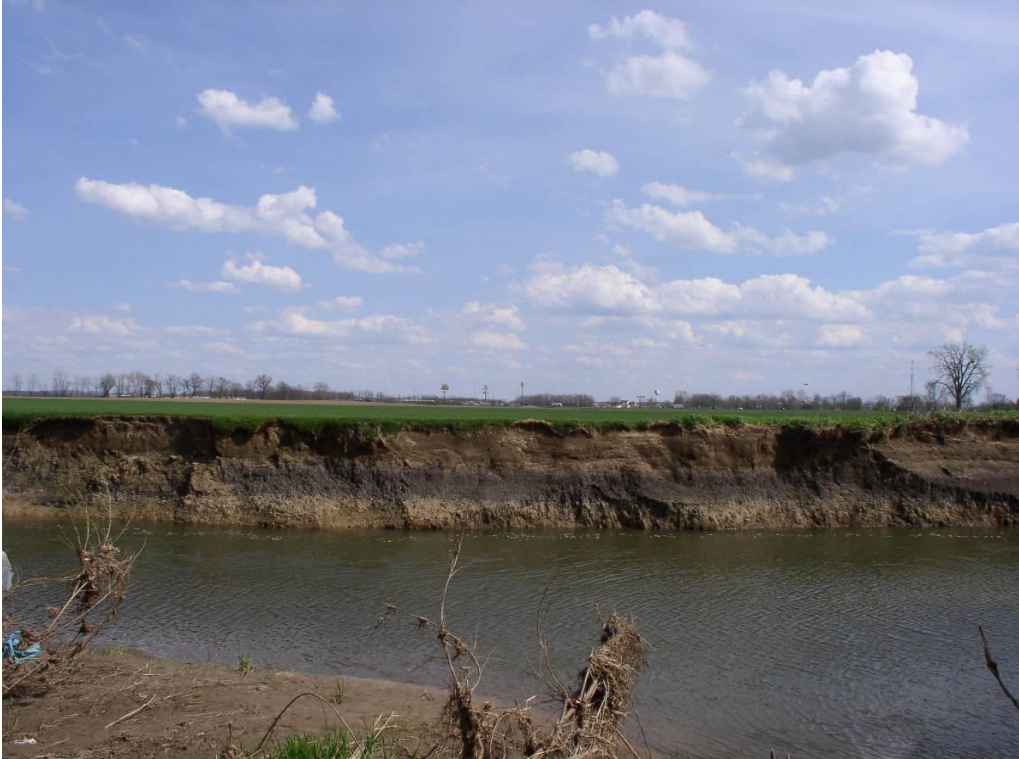
Figure 3 Licking River bank failure in the flood pool
