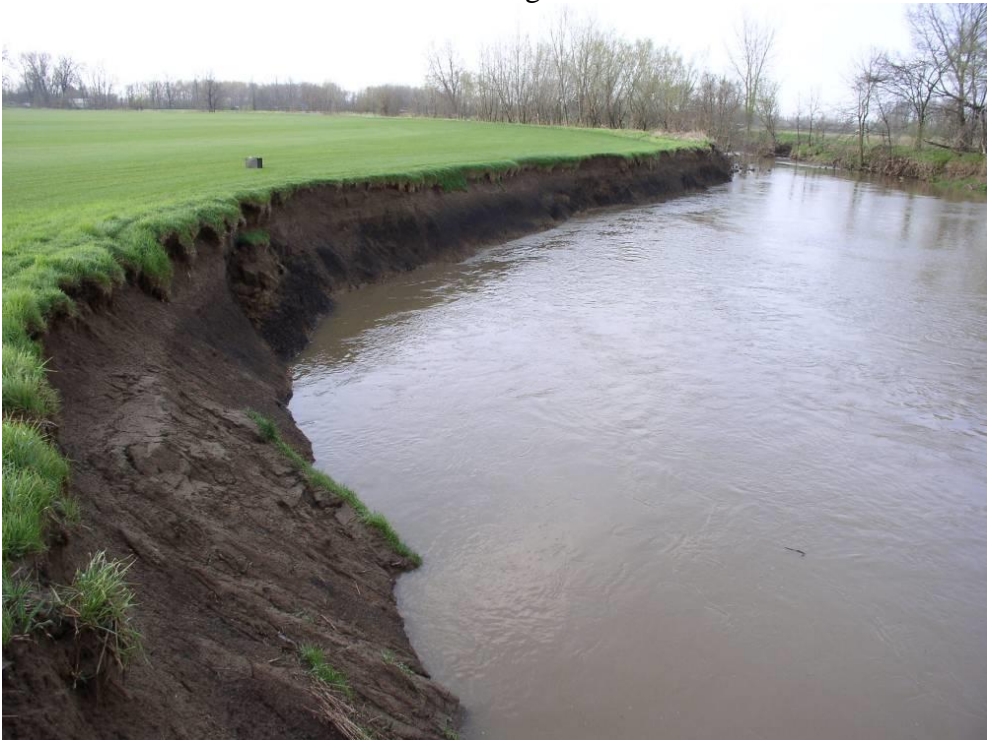
Figure 6. Dramatic bank failure along the Licking River in the proposed flood pool.
